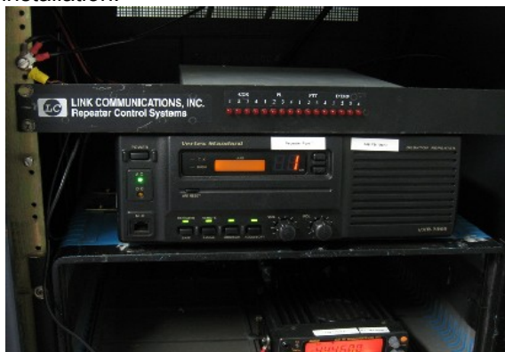
VHF repeater and controller at Kulani
