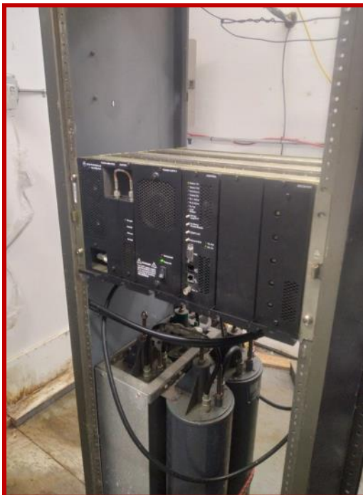
The actual VHF repeater, with duplexers below.
